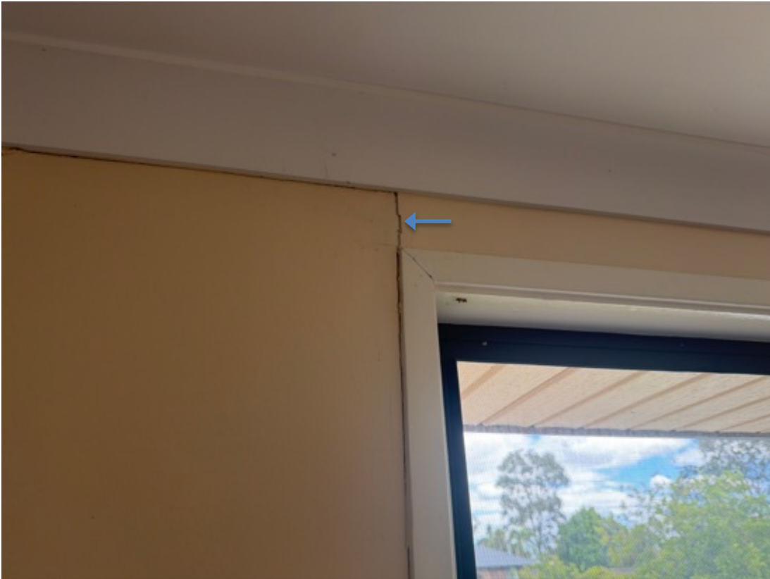
Bedroom plasterboard and cornices display cracking, front mid section bedroom example above.
