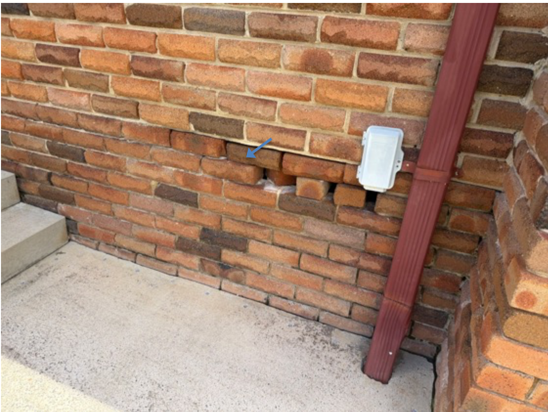
Sections of external brickwork displays salt attack and rising damp, front elevation example above.
