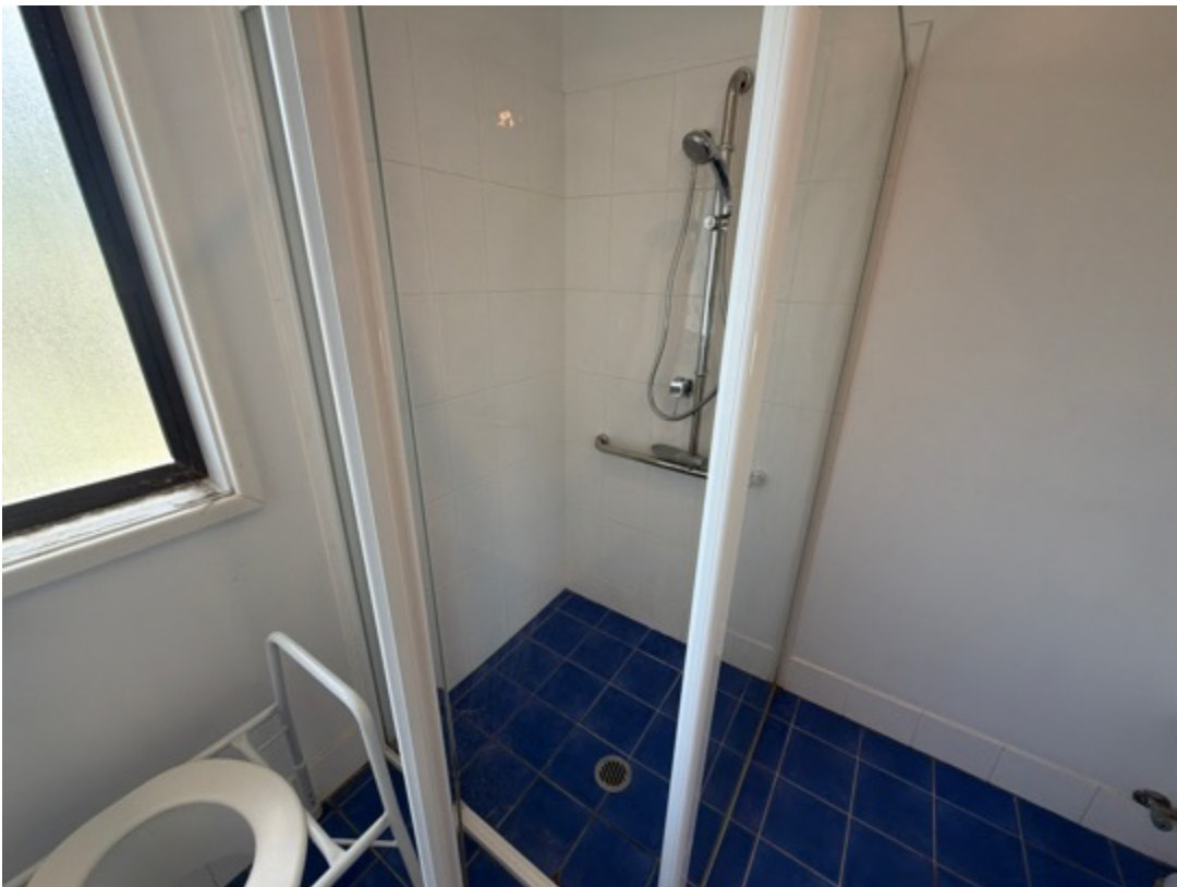
Water pressure tested, is sufficient.
