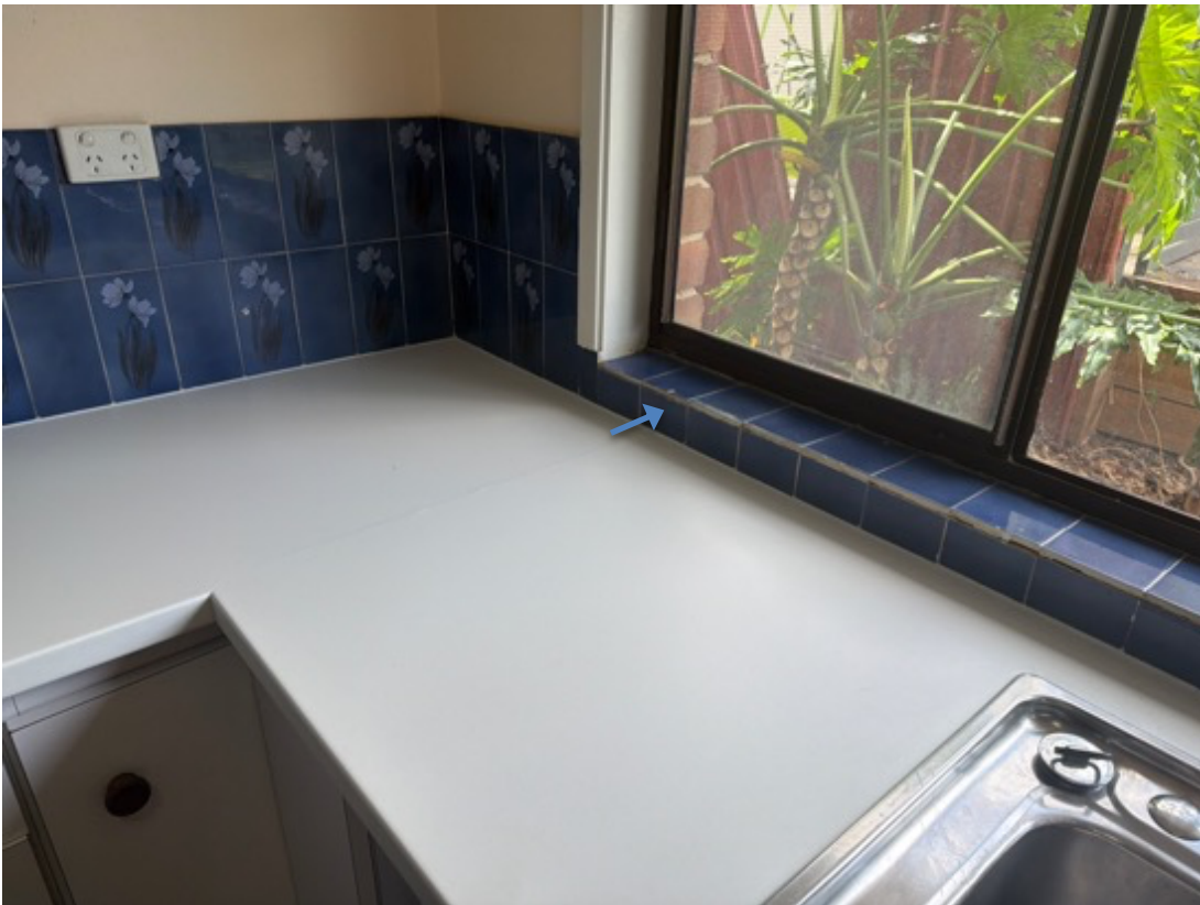
Sections of kitchen tiles are cracked and chipped, consistent with age.
