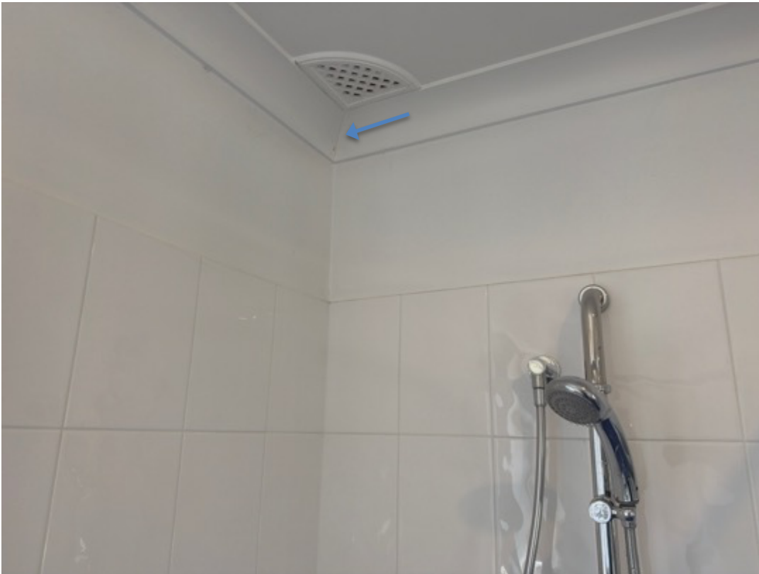
Sections of internal plasterboard and cornices display hairline cracking, example above the bathroom shower.
