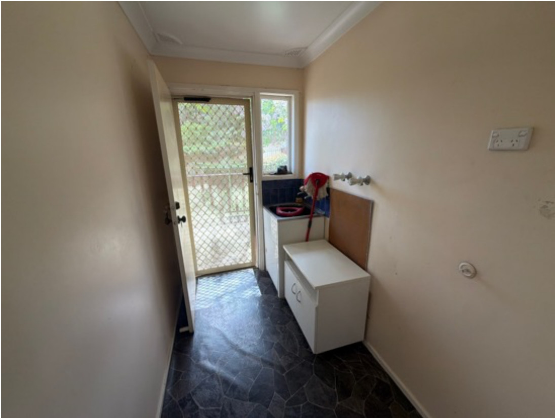
The laundry walls display signs of pest damage, refer to pest report.
