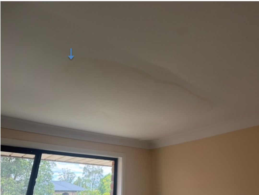
The front facing bedroom ceiling is water stained here.
