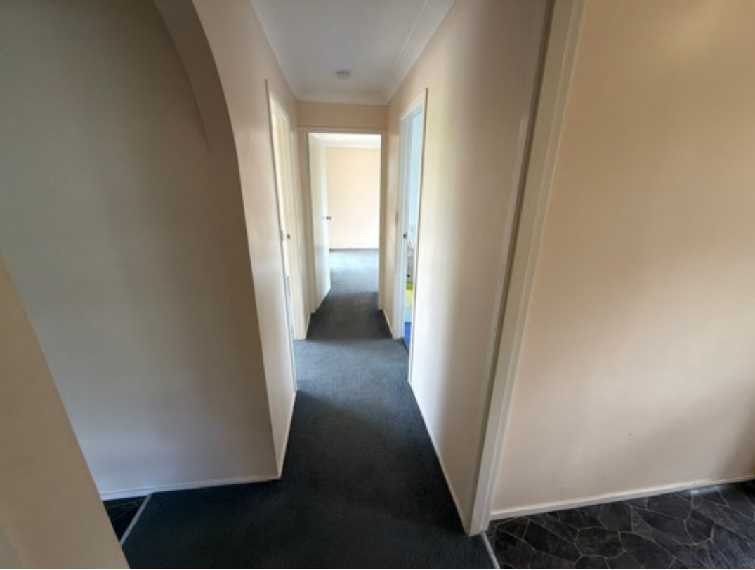
Bedroom floors and doorways are termite affected.
