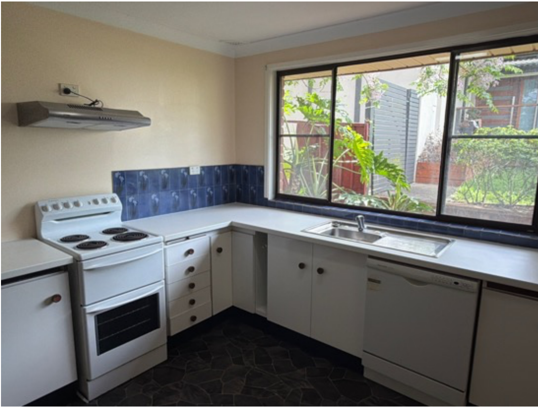
Water pressure tested, is sufficient.
