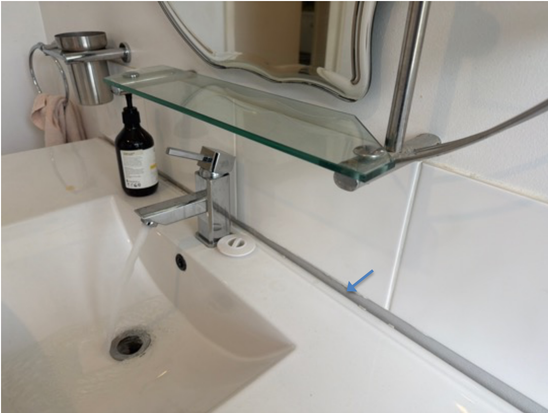
The vanity has separation away from splashback tiles.
